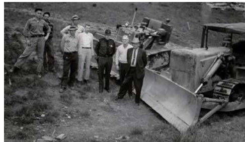
Construction begins with a pair of borrowed bulldozers, 1948; the only person identified in this photo is Sgt. Ralph D. Trumbo (center). Images in this article are courtesy of the West Virginia State Police Academy Archives, Institute unless otherwise noted.
